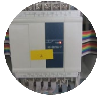
PLC (Made In Taiwan)
